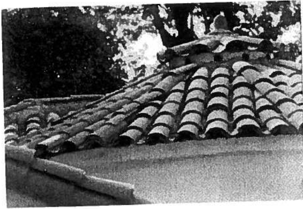
Photograph above shows Two-Piece Red-Clay Barrel Mission Tile at 4648 Ladera Lane. Below is historic one-piece "S" Mission Tile located at 4651 Ladera Lane.
