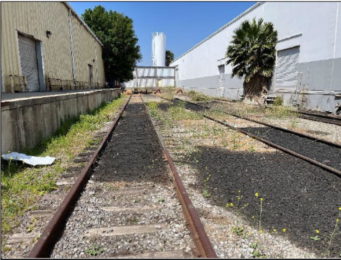
15. Evidence of Surface Staining at the Western Portion of the Railroad Spur
