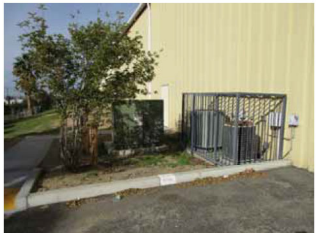
12. View of the transformer located on the south side of the building (1151 Palmyrita Avenue), view facing west.
