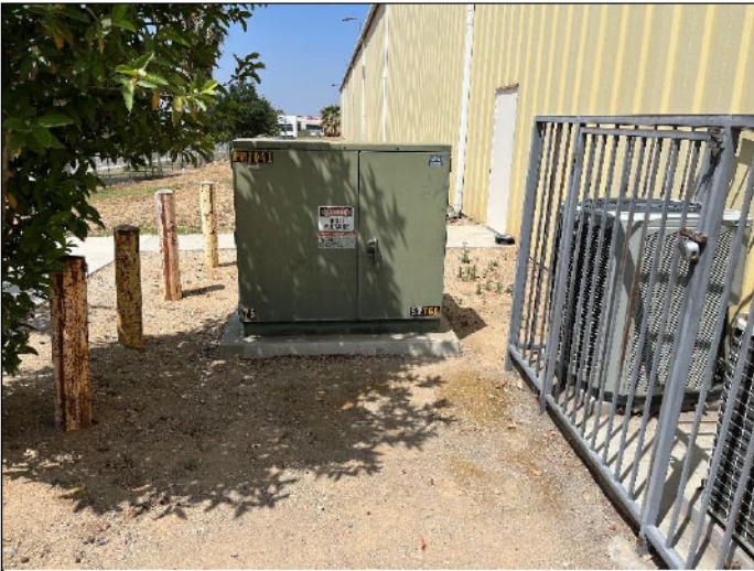
11. SCE Pad-Mounted Electrical Transformer
