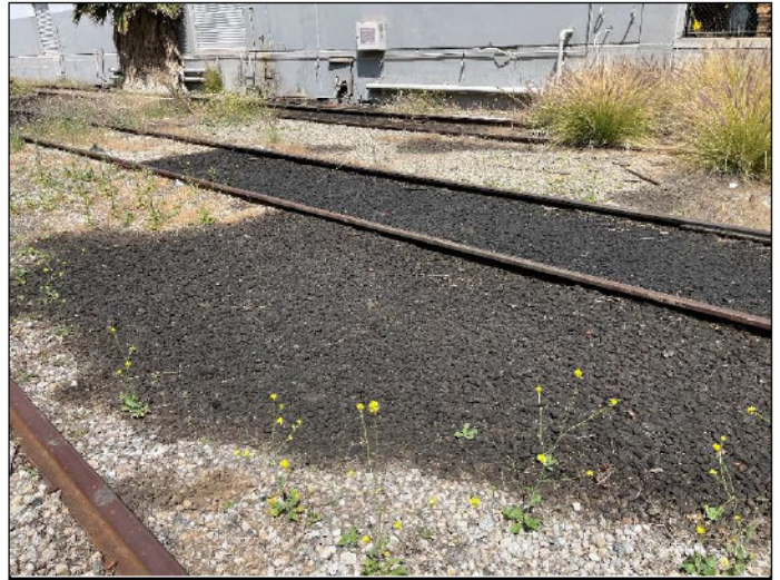
16. Surface Staining at the Western Portion of the Railroad Spur
