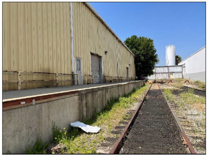
14. Western Portion of the Railroad Spur (surface staining)
