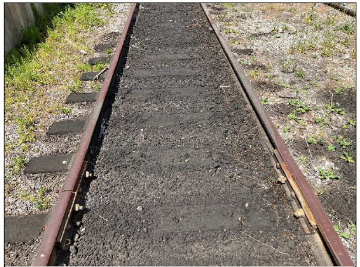
18. Surface Staining at the Western Portion of the Railroad Spur
