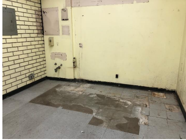
8. View of former maintenance area on the ground level of the retail structure.
