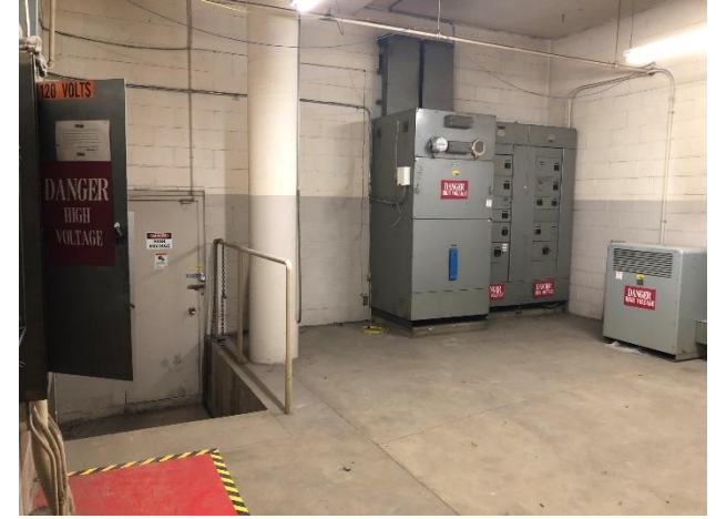
15. View of electrical equipment room in the retail structure basement level.
