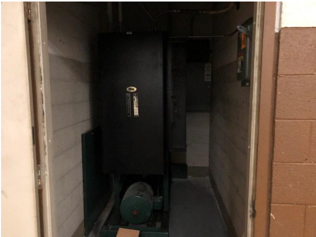
16. View of freight elevator equipment room in the retail structure basement level.
