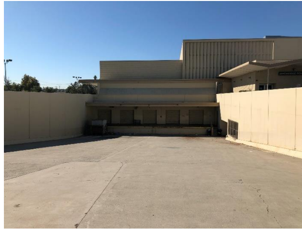
2. View of loading dock on the northern side of the retail structure.
