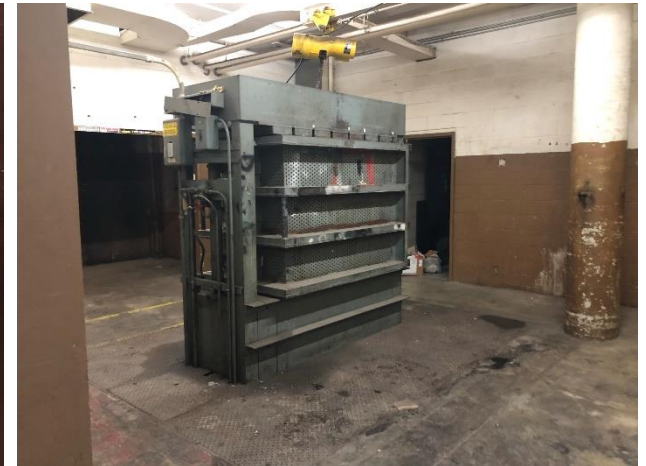
18. View of trash compactor in the retail structure basement level.
