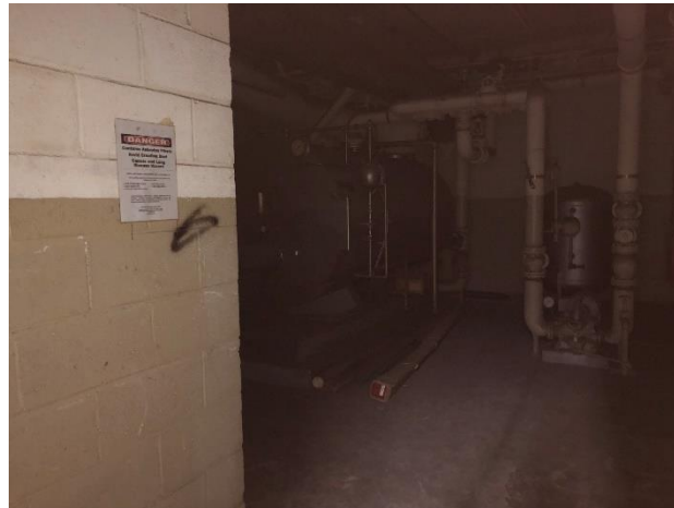
17. View of disconnected boiler in the retail structure basement level.
